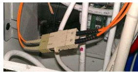
Fiber optic cable
